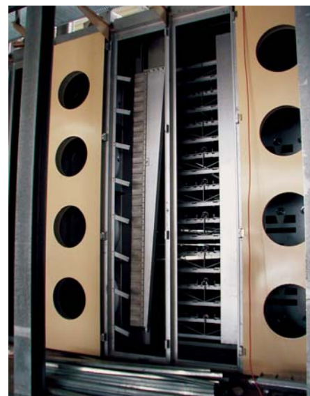
Fig. 6: Linnox burner mounted in the gypsum and fiber board dryer
