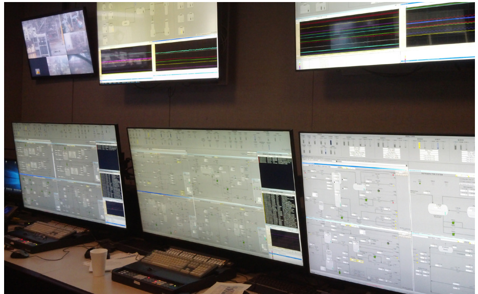
Chevron Oronite seeks to manage the lifecycle of its existing automation assets while employing new digital technologies.
