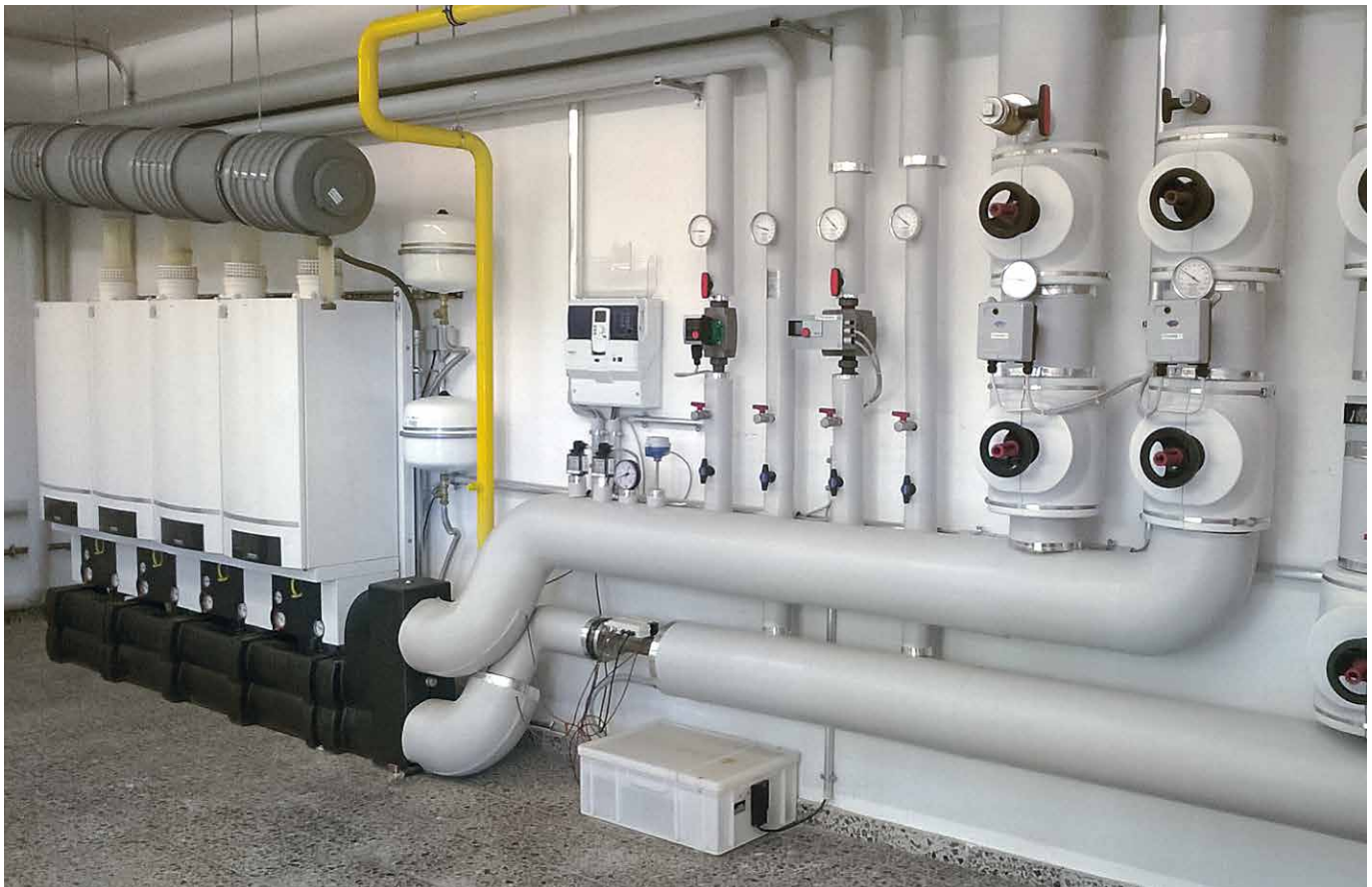
Preheating system with four condensing boilers and speed-controlled circulation pumps
