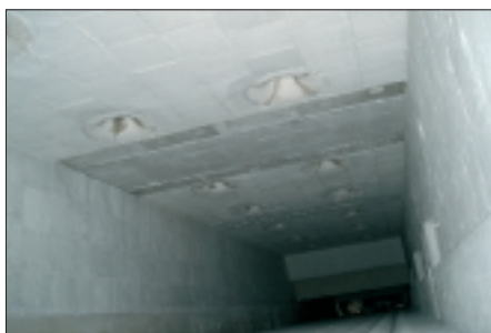
Fig. 1: Interior view of a lifting hearth furnace with flat flame burner quarts in the roof
