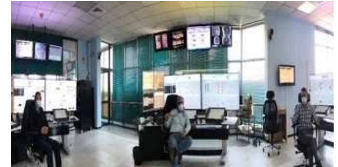
Control Room at Anglo American
