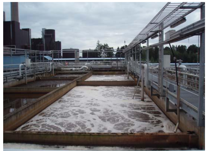
Espoon Vesi’s water treatment plant utilizes Honeywell’s remote network services to help ensure clean water production and distribution.
