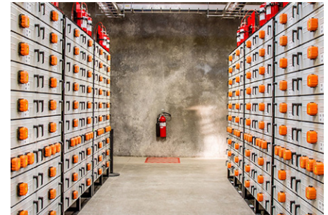
Figure 3: Honeywell's BESS platform, along with remote operations systems and the Experion Energy Control System, enables automated and agile renewable energy operations.
